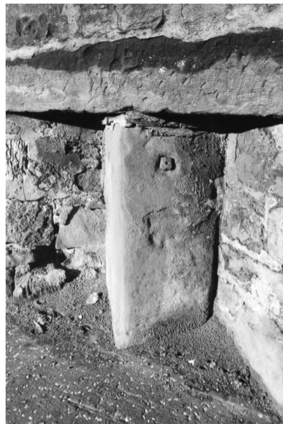
Figure 8: Type E, showing as a triangular plan, post restoration, in Slateford Road (photo by Adrian Summer).
