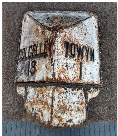
Damaged milepost 7/03/22 Photo: Hilary Jones
