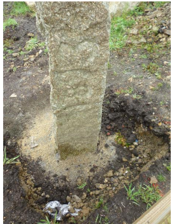
Figure 16: SX136736 A30 Temple Moor. Restored fingerpost packed with sand in a heavy concrete base.
