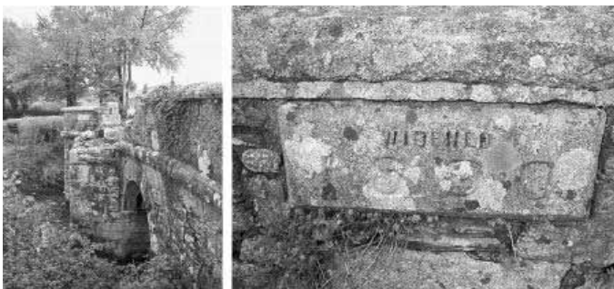
Figs 10 & 11 Berrio Bridge at SX273756 and the bridge widening commemorative stone. Recent traffic damage missed the date stone by inches
